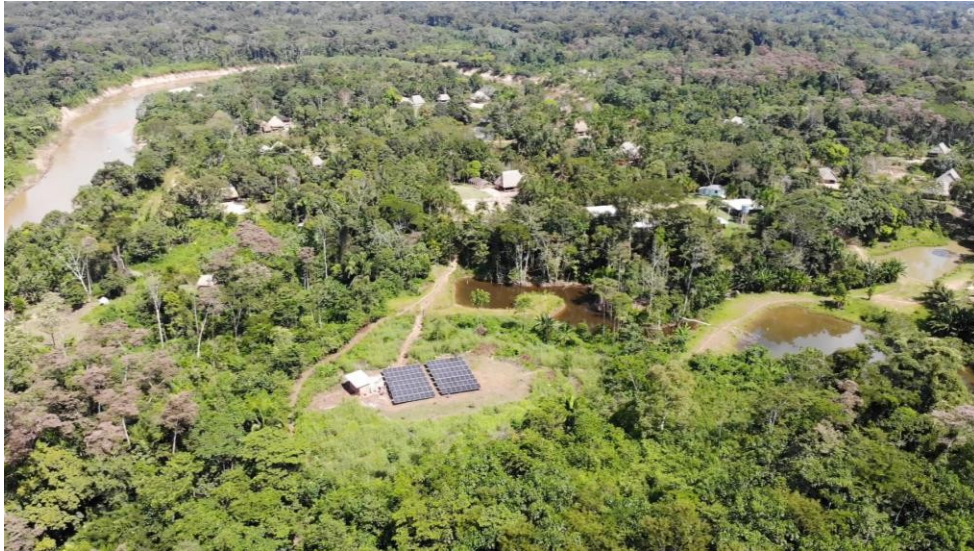
Figure 3: Off-grid solar energy system installed 20 .
